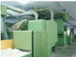
Blow Room: LR – 1993
